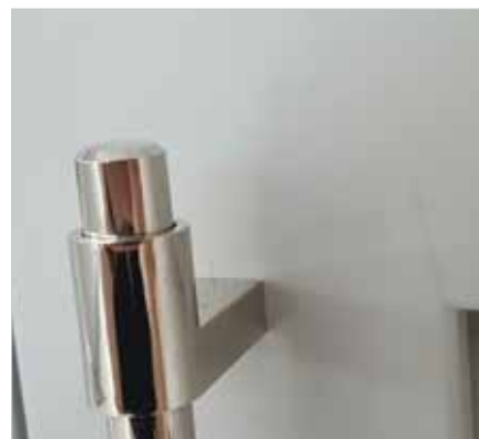
The whisper line does not follow the line of the joint.
