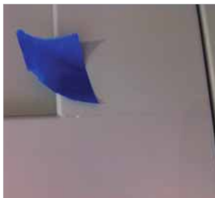
The whisper line has formed but caused the paint to flake off the surface of the door.
