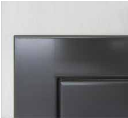
The shadow of the joint is visible underneath the finished top coat. Paint unbroken.
